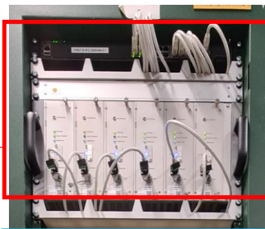
CROME Rack at EHN1 (North Area)
